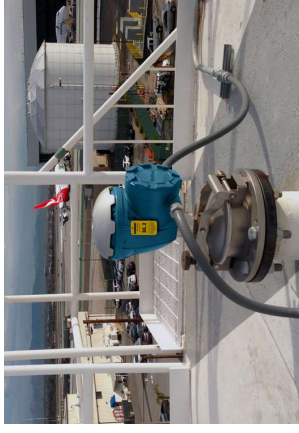
Figure 2.10: Modern radar level gauge on a fixed roof tank.
