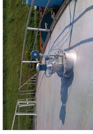
Figure 3.4: Manways are normally located near the tank wall which provides mechanical stability.
